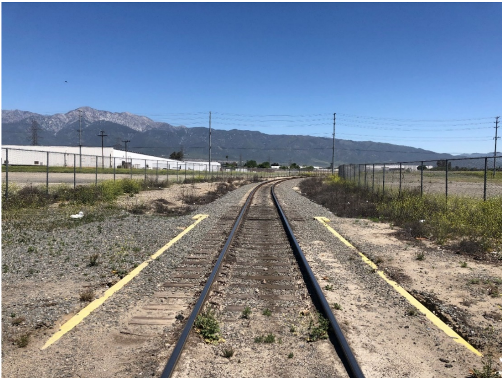
Figure 5-2 View of railroad tracks bisecting the Project area, view of the north
