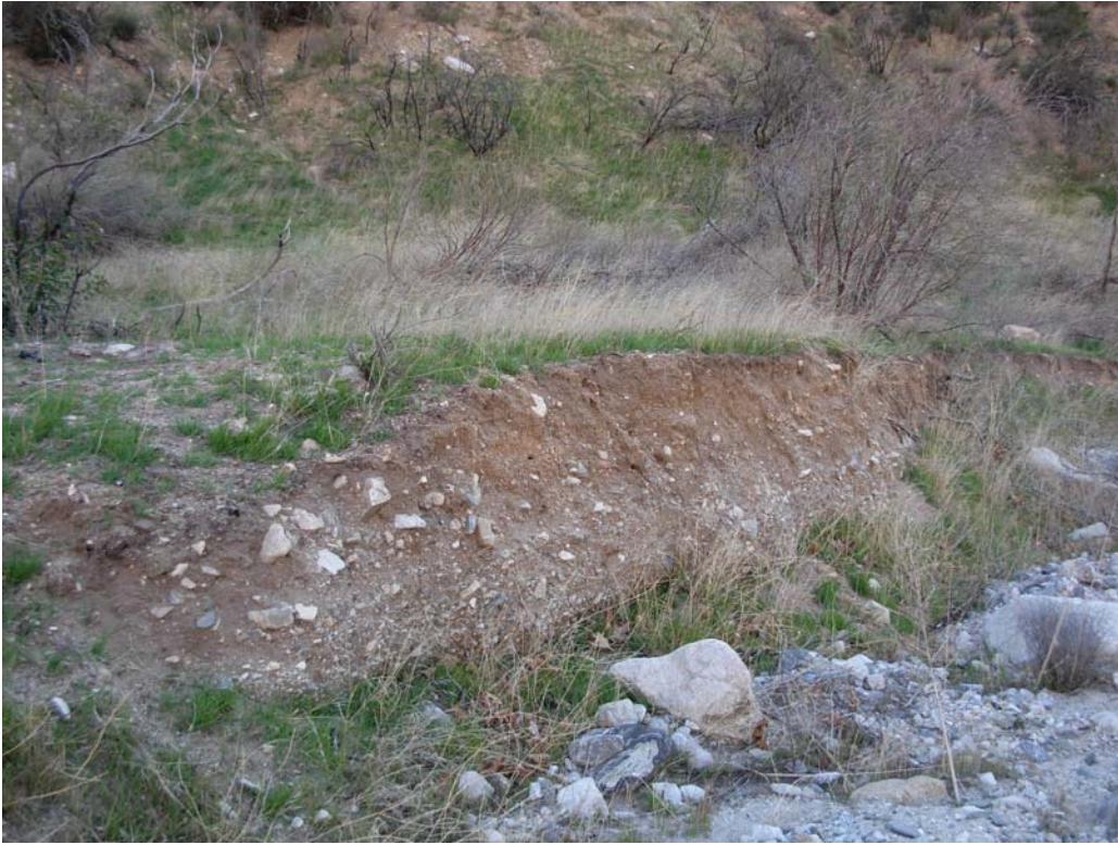
Photo 22: Scouring on East Bank of Tributary 5
